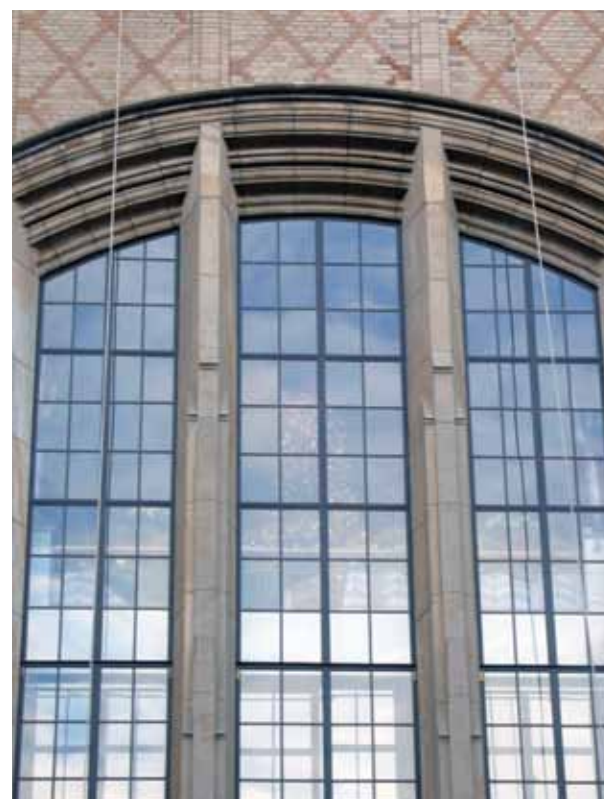
The restored steel windows at Columbia University Hospital now greet visitors as they enter the medical complex. Many viewers thought they were new. Photo: Richard MacDowell, Grenadier Corp.
